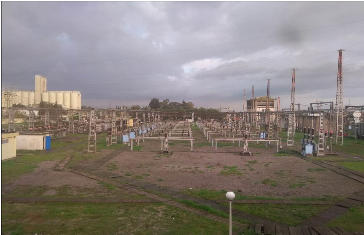
Figure 3.1. Poste 220/90/60/30kV EL HADJAR [54].
